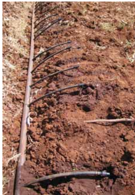
Main pipe supplies the drip water
